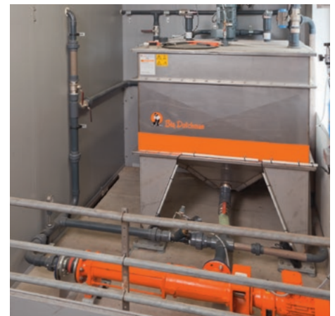
Storage tank to supply CallMatic pro
