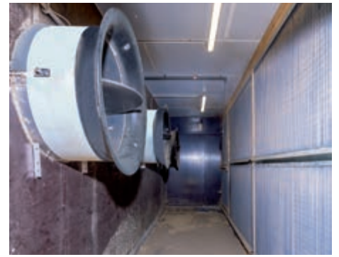
Pressure corridor with upstream StuffNix dust filter
