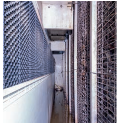
On the left: droplet separator, on the right: biological filter bank with brushwood filling
