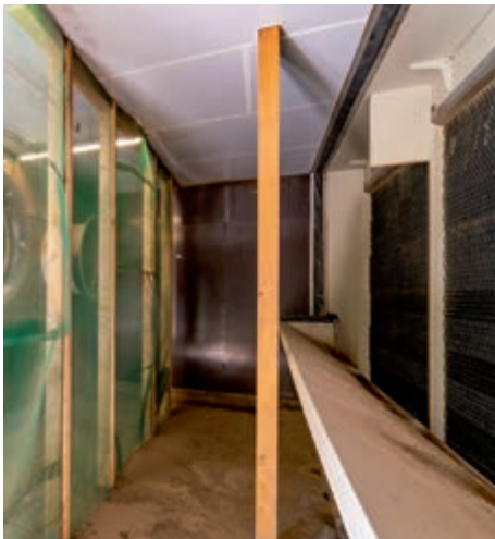
Fans push the exhaust air through the filter bank; an impact net ensures good distribution of the air
