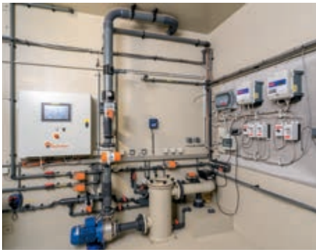
Pre-installed technical room with control box
