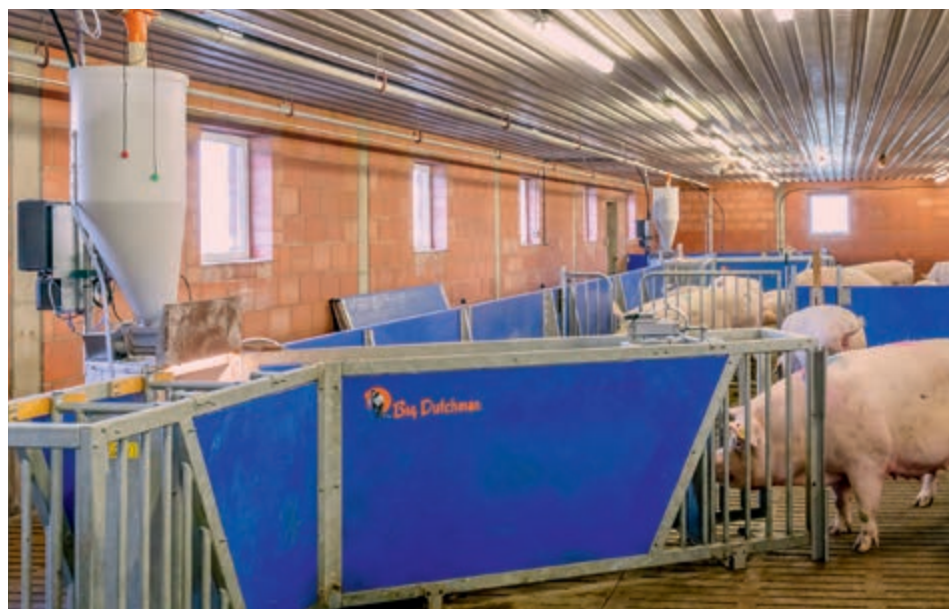
Use of a DiffAir ceiling in a gestation house for sows
