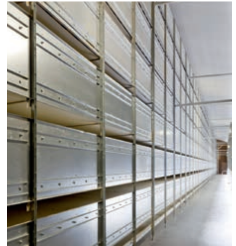
Air exit side
