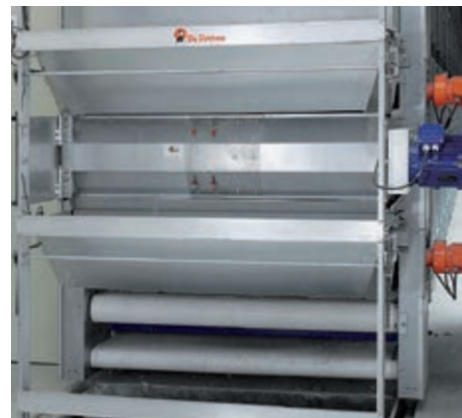
Chopper installed between tiers 3 and 4
