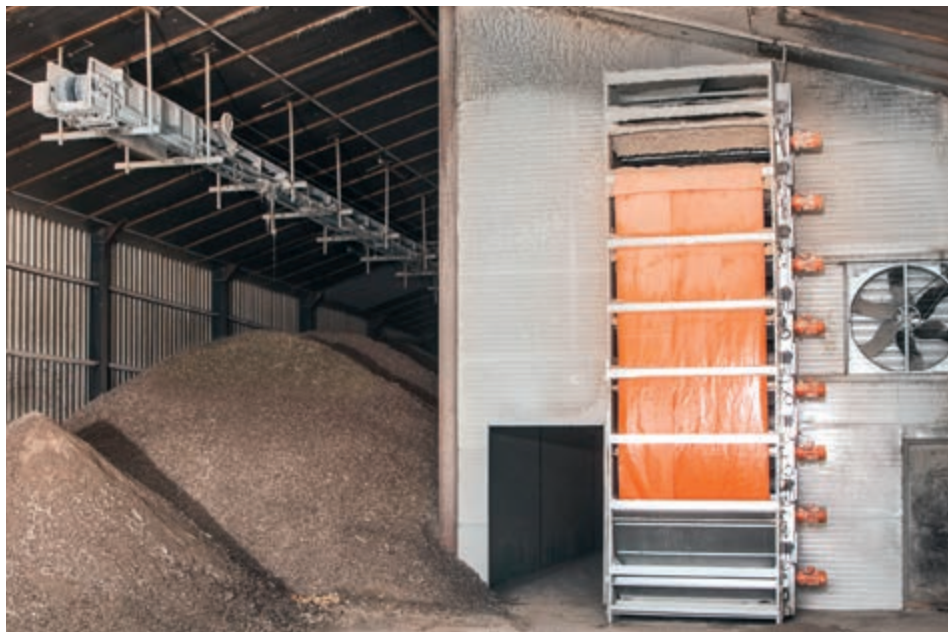
OptiSec and manure storage in the same building
