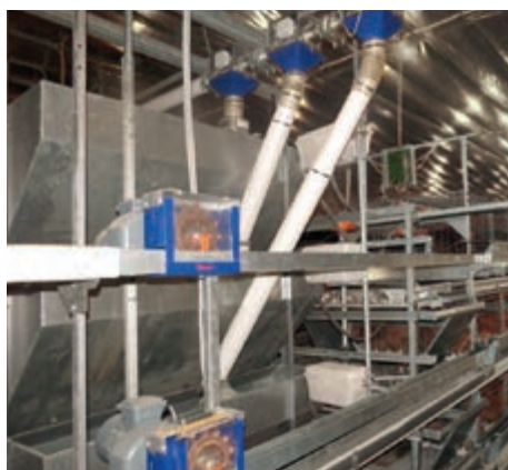
Feed hoppers in each tier are supplied with an exactly defined feed quantity via one feed valve each
