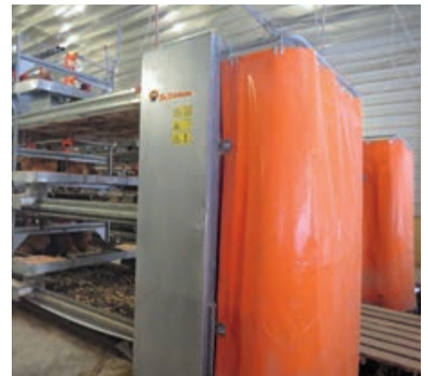
Plastic curtain in front of the manure chute
