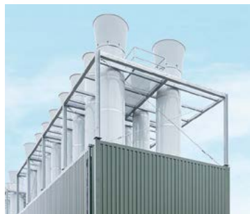
Ventilation, heating, cooling
