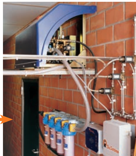
Central pump unit with four filters
