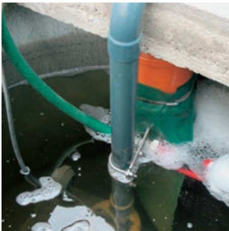
Use of a submersible pump to supply water to CoolBox
