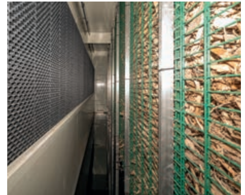
View into the second pressure chamber: droplet separator (left), biological filter bank (right)
