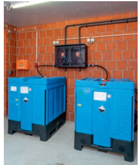
Acid and alkali dosing
