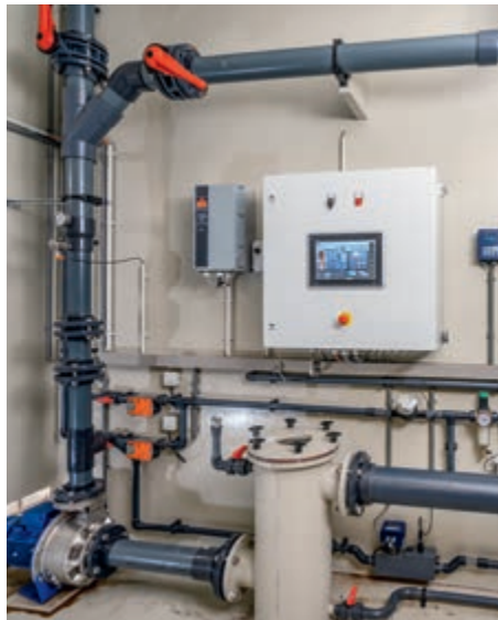
Pre-installed technical room with control box
