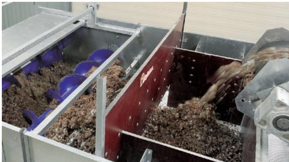
The distributing augers fill the belts evenly
