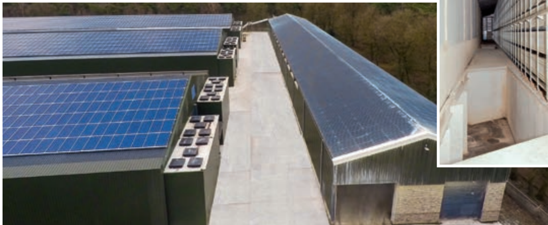
Cost-efficient solution: one OptiSec for three layer houses with 90,000 layers each; the air reaches the dryer underground
