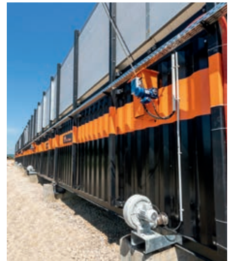
A compressor forces fresh air into the material to be composted
