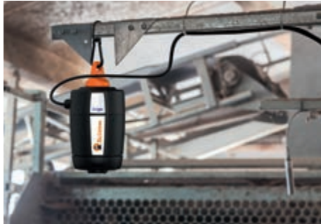
NH 3 measuring at an OptiSec dryer
